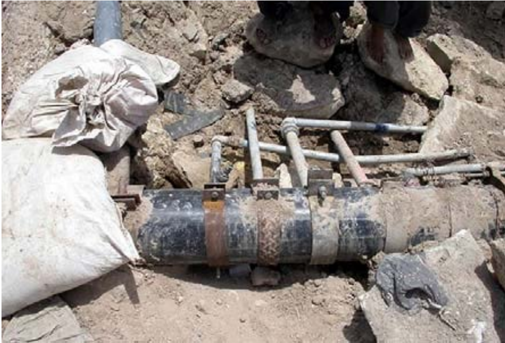
Figure 34. Illegal taps in the distribution lines, Nassiriya, Iraq (SIGIR 2010).
